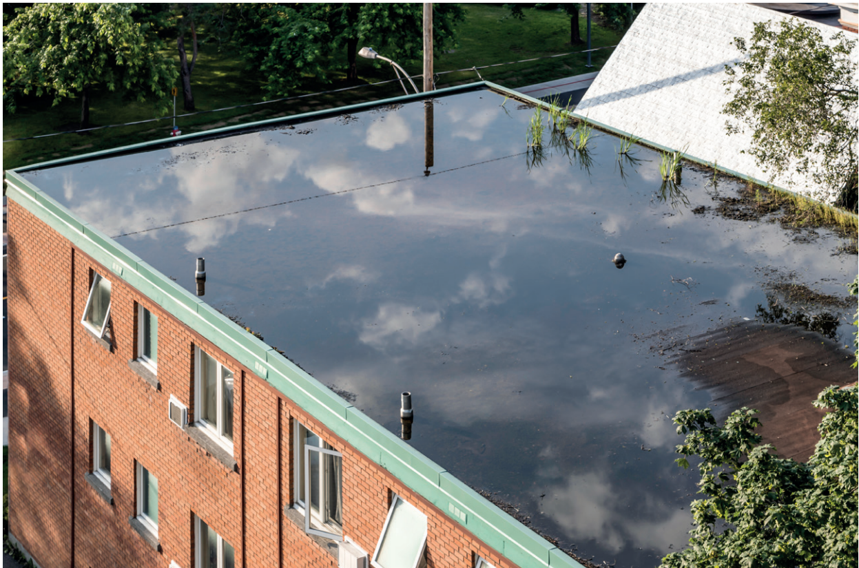
Figure 1: Ponding on a typical flat roof
